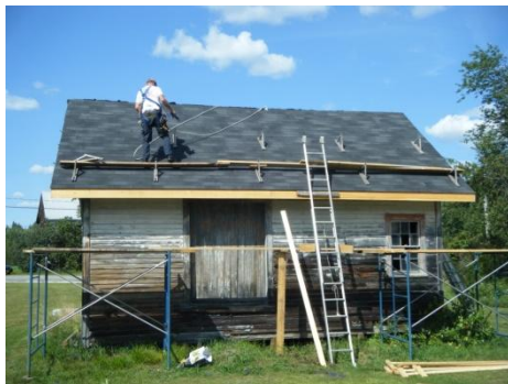
Director Richard Hatch shingling no doubt glad to finally reach the rear roof peak!
